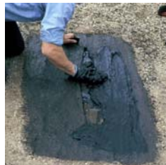
PRIOR TO REPAIRS
