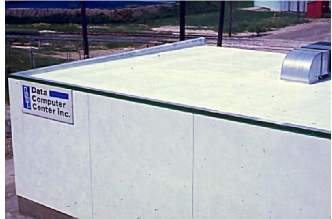
SWEPACO White Roof Shield enhances the appearance of any building ... while it insulates and protects the roof.
